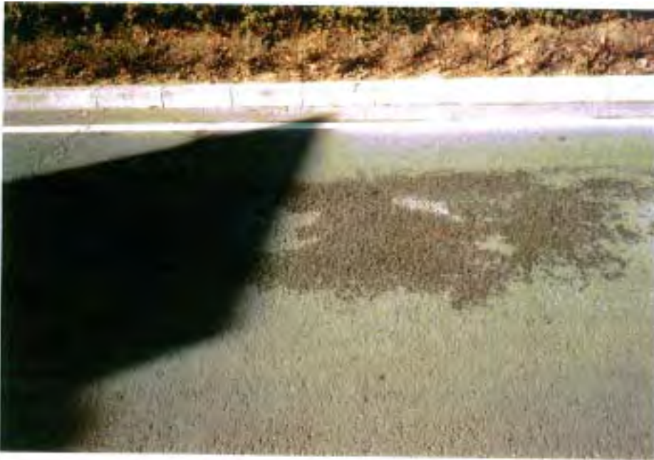
Aggregate Scattering Spots End of Inspected Opposite Lane
